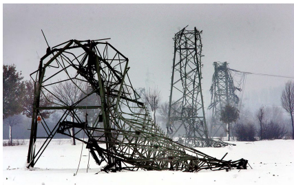
Figure: Destroyed power lines in winter 2005; photo: Jürgen Peperhowe
